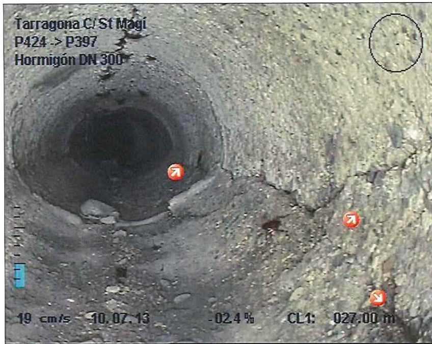
Foto: 6_7B, MPEG #: 110713_1, 00:02:36 26,5m, ROTURA PUNTUAL
